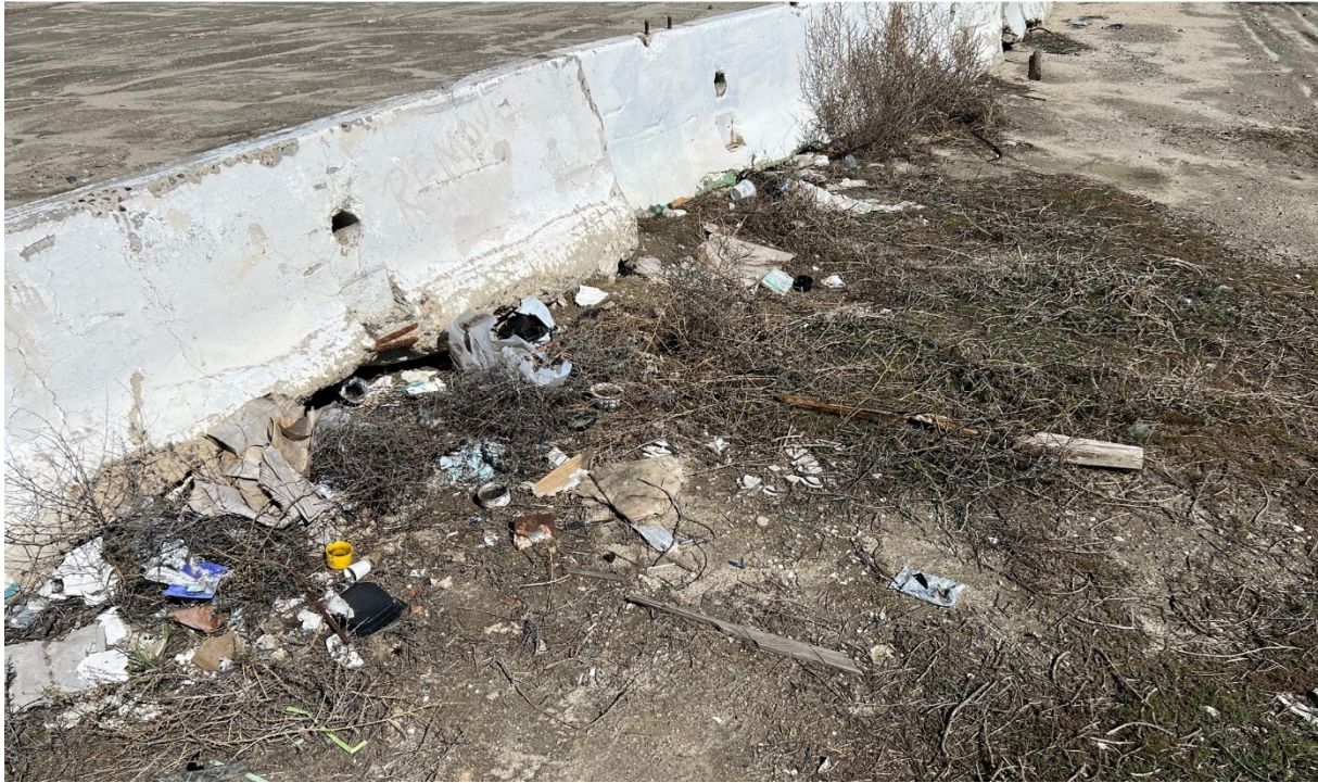
Closer view of trash accumulations near barriers along northern barrier of the northern property.
